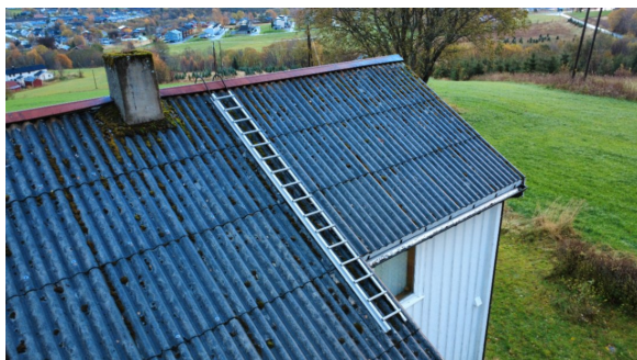
Pusset pipe mangler pipehatt
