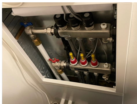
Sentral for gulvvarmen
