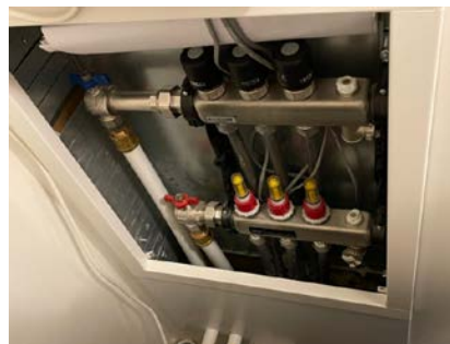
Sentral for gulvvarmen
