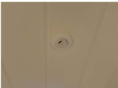
Sprinkelhode i himling.
