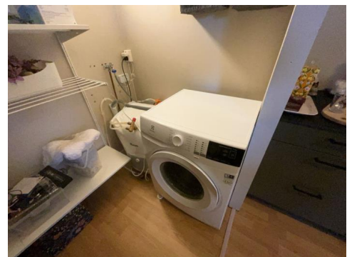
Opplegg for vaskemaskin.
