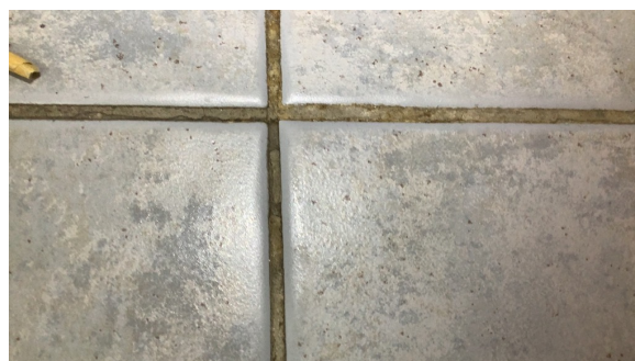
Riss i flisfuge.
