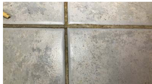
Riss i flisfuge.
