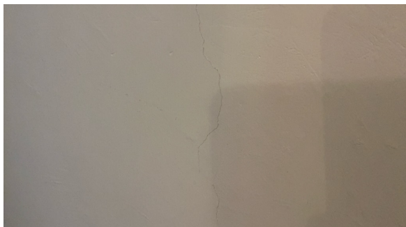
Riss i pipe
