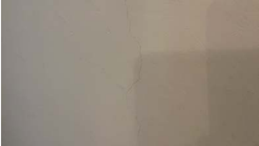
Riss i pipe
