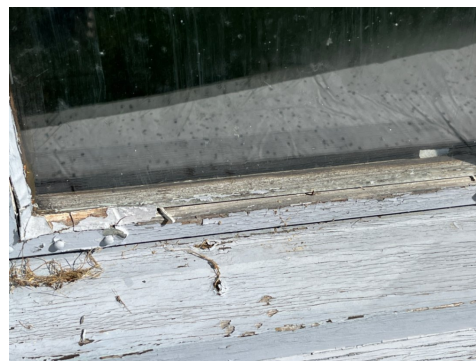
Værslitt, manglende kitt rundt glass.
