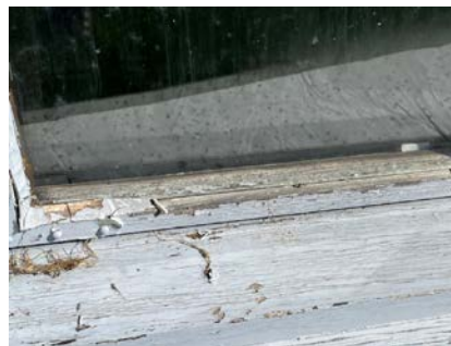
Værslitt, manglende kitt rundt glass.
