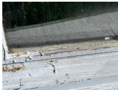
Værslitt, manglende kitt rundt glass.
