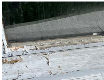
Værslitt, manglende kitt rundt glass.
