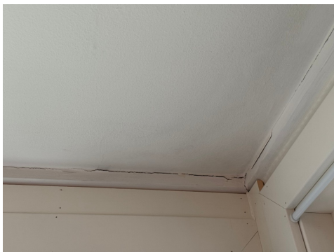
Sprekk i overgang list - himling.
