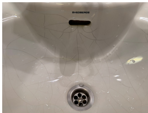
Riss/krakelering i servant.
