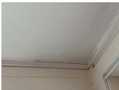
Sprekke i overgang list - himling.
