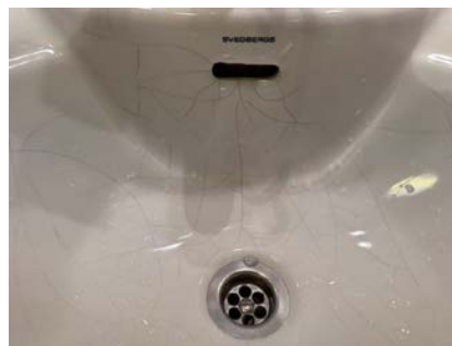
Riss/krakelering i servant.
