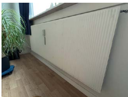
Eldre radiatorovn i stue.
