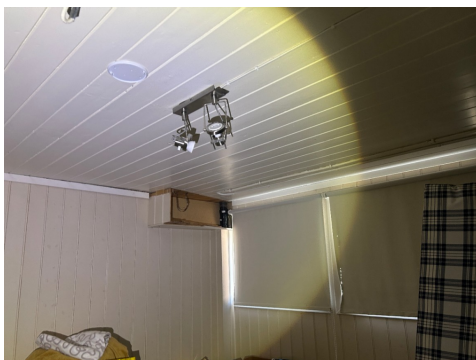
Brekkasje/skade i himling.
