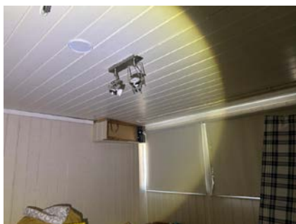
Brekasje/skade i himling.
