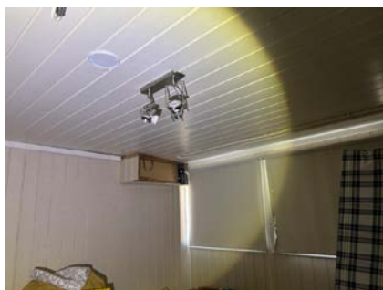
Brekasje/skade i himling.
