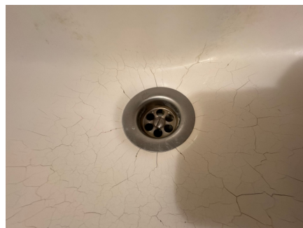
Riss/sprekker i servanten.
