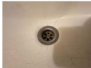
Riss/sprekker i servanten.
