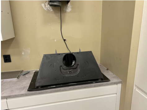
Ventilator tatt ned.
