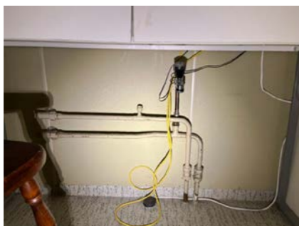
Opplegg for vaskemaskin.
