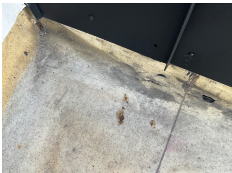
Hull, skade i belegg
