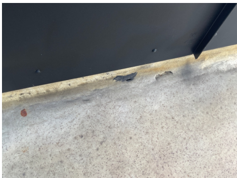
Hull, skade i belegg
