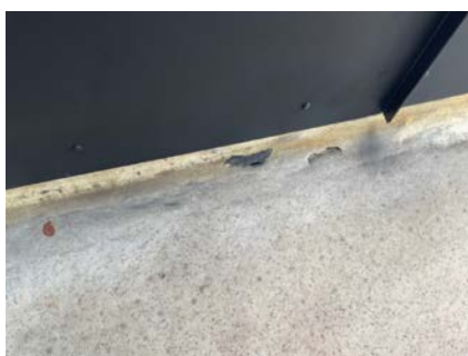
Hull, skade i belegg
