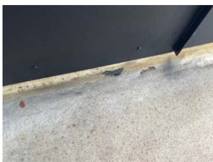
Hull, skade i belegg
