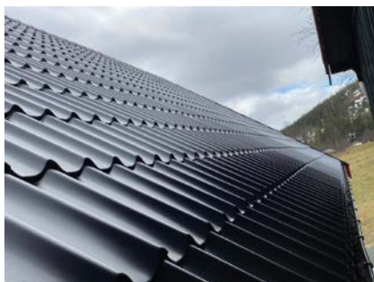
Bulker/rust i plater.
