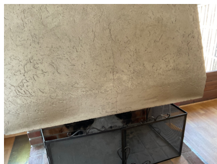
Overflate-riss i peiskappe.
