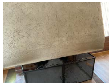
Overflate-riss i peiskappe.
