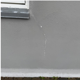
Riss i mur under vindu vegg vest.
