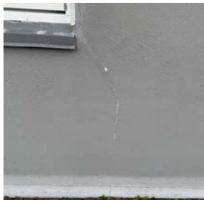
Riss i mur under vindu vegg vest.
