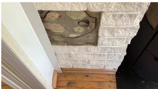
Manglende ildfast plate under sotluke.
