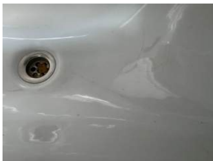
Riss/sprekke i servant.
