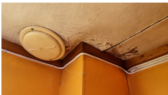
Fuktskader i himling.
