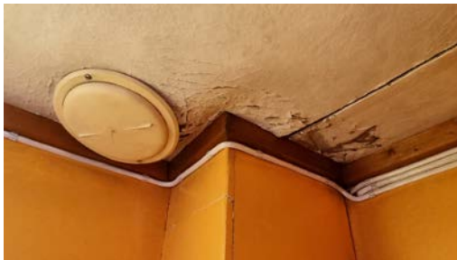
Fuktskader i himling.
