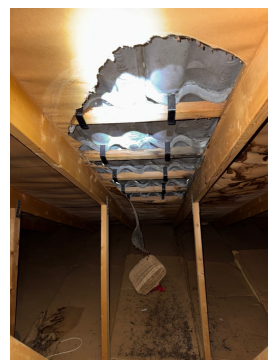
Store hull/manglende undertak
