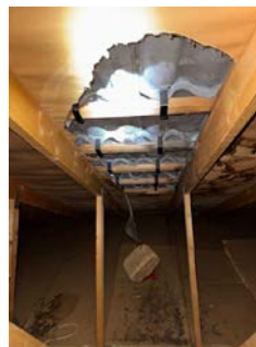
Store hull/manglende undertak
