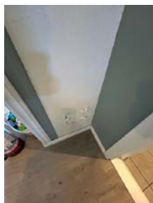
Manglende ubrennbar plate under feieluke.
