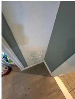
Manglende ubrennbar plate under feieluke.
