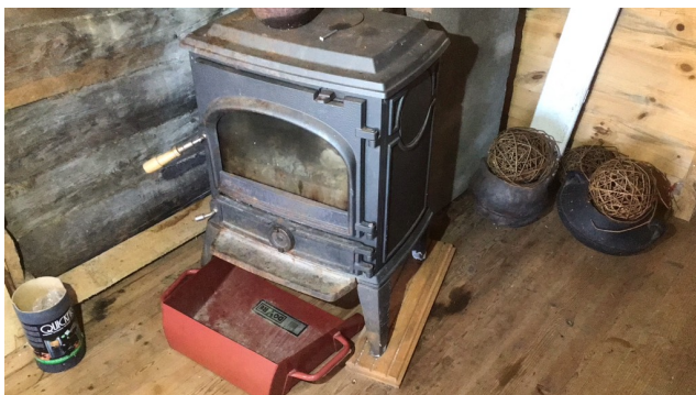
Mangler ildfast plate under ovnen
