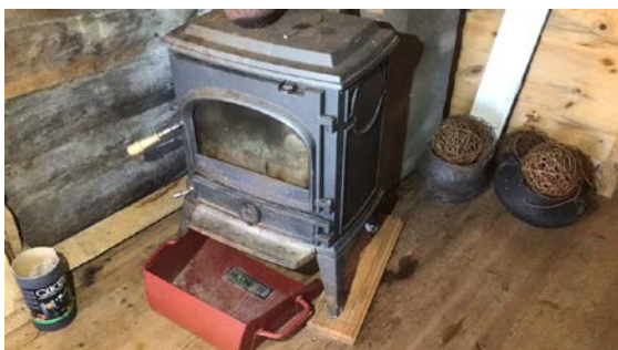
Mangler ildfast plate under ovnen
