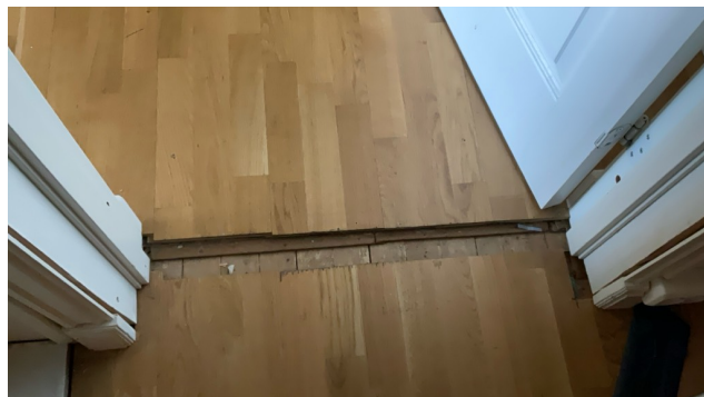
Det mangler overgangslister.
