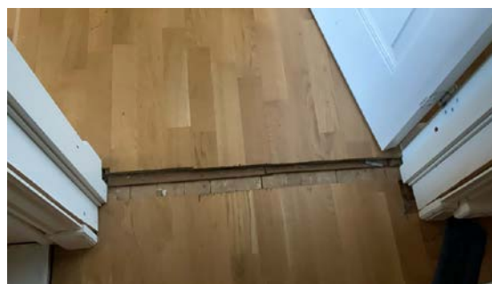
Det mangler overgangslist.
