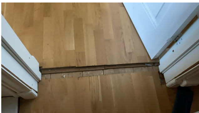
Det mangler overgangslister.
