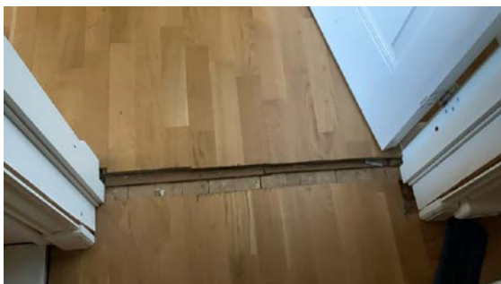
Det mangler overgangslist.
