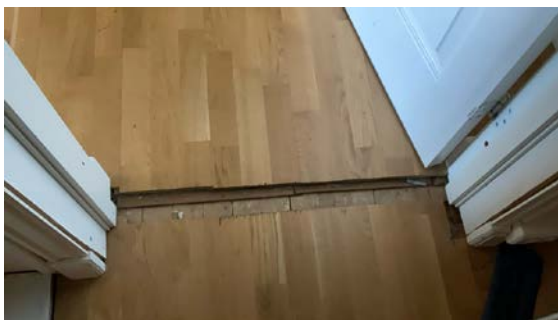
Det mangler overgangslist.
