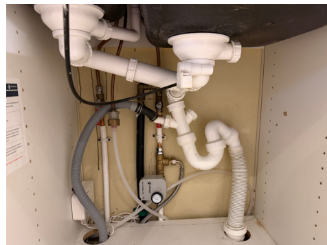
Røropplegg under vask.
