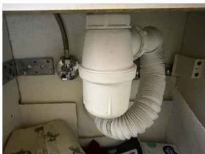
Røropplegg under servant.
