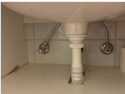
Røropplegg under servant.
