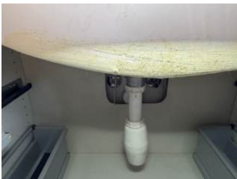
Røropplegg under servant.
