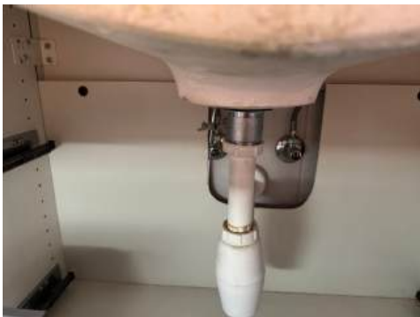
Røropplegg under servant.
