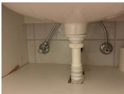
Røropplegg under servant.
