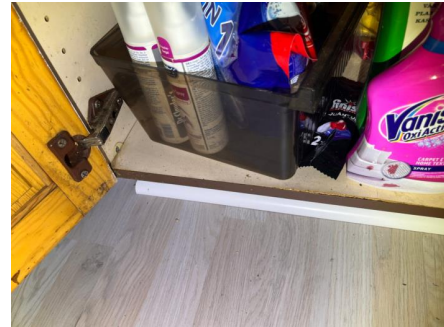
Fuktsvelling i bunnplate
